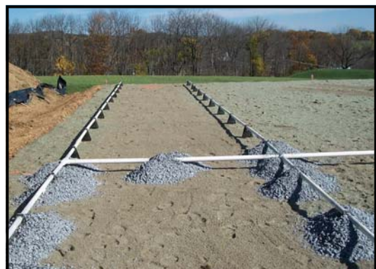
Large Pressurized Drain Stone Field
